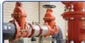
Watt's Fire Suppression Valves
