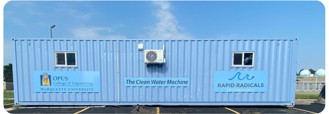
Fig. 3: Pilot-Scale System at Milwaukee Treatment Plant
